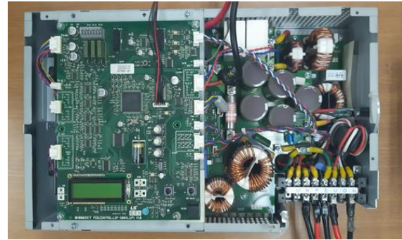
Fig. 9. PV power conditioning system(PCS) of 4 kW.
