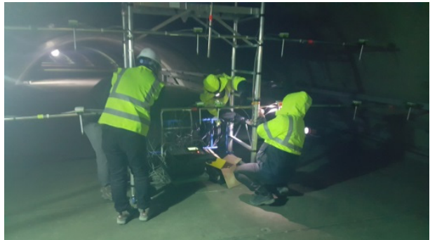
Fig. 4. Sensor installation overview
