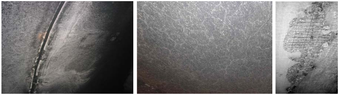
Fig. 16. Damaged surface by fire on subway (left) and road (middle), tauern (right)
