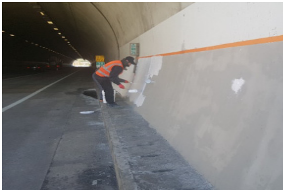
(c) Installation Instrument
