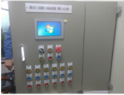
(a)관수제어시스템 외부 (a)Integrated system outside
