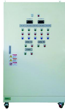
Fig. 6. Control panel of gastight shutoff valve
