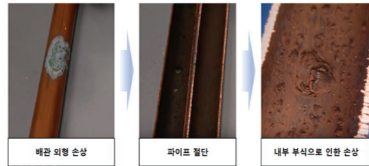
Fig. 7 Pipe line damage status
