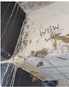
(a) Bond failure at S-2
