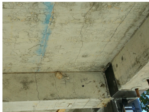
(b) Flexural crack at S-2
