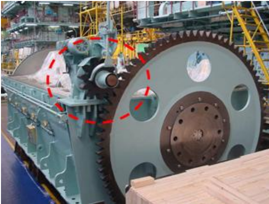
(a) Turning gear and flywheel
