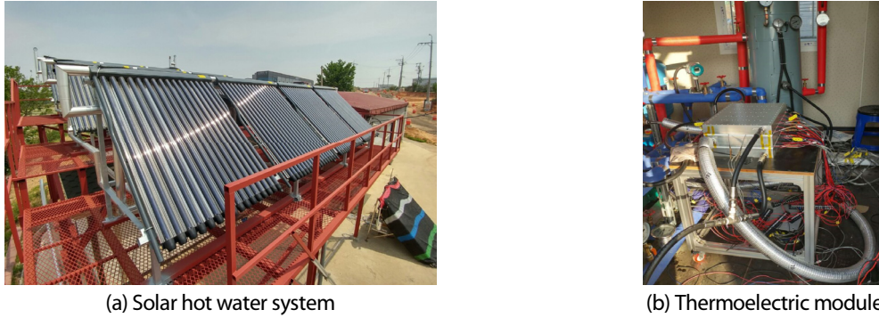
Fig. 6 Picture of solar hot water system and thermoelectric module installed in control room
