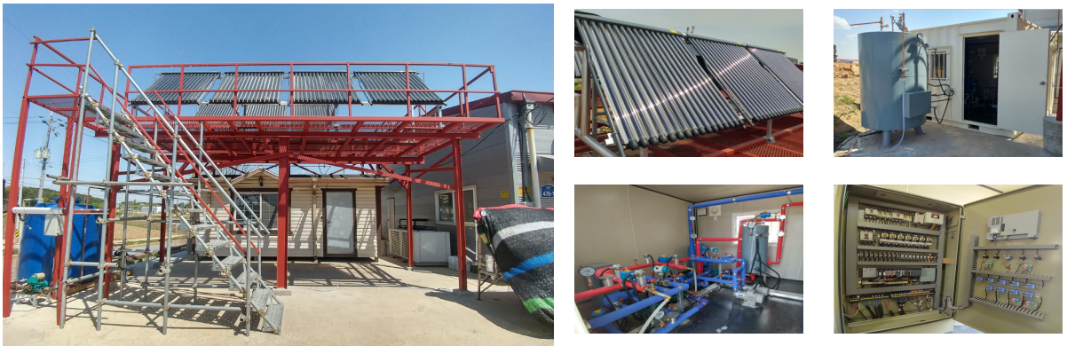
Fig. 3 Double vacuum type solar hot water system
