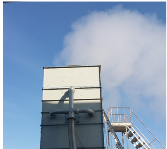
Fig. 3. Cooling tower of plume phenomenon
