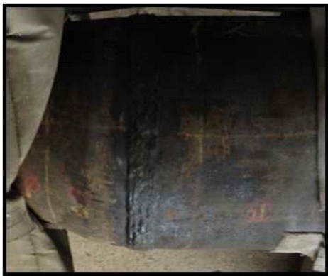
Fig. 2. Damaged reducer in RHDS process.
