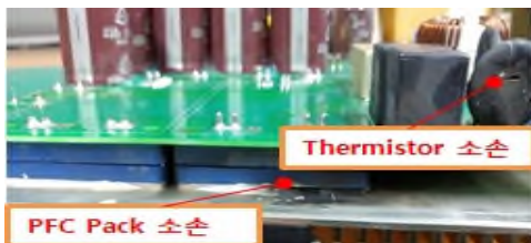
Fig. 4. PFC pack and thermistor burnout due to 1-wire ground fault
