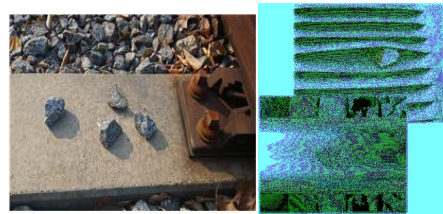
Fig. 1. Damage of track facilities due to scattering of railway ballast on the sleepers
