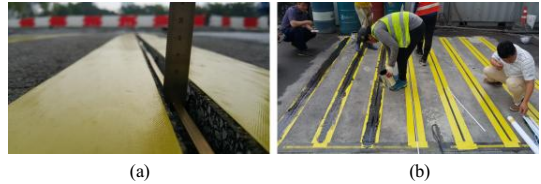
Fig. 8. Traffic sensor installation 2 nd stage (a) Attached the sensor (b) placing the resin
