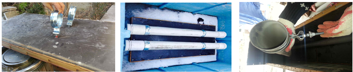
a. Production of Fixing Device b. Hollow Core Materials and Form c. The details of Fixing Device
