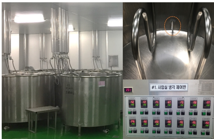
Figure 1. Fermentation tanks and controllers (left), Temperature sensor inside a fermentation tank (upper right), and control panel for controlling temperature of a fermentation tank based on the temperature sensor (lower right)
