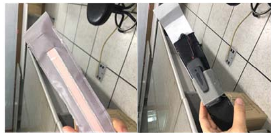
<Fig. 20> Inverter inserted into the back of luminous device. Photographed by the author. (December 17, 2016).
