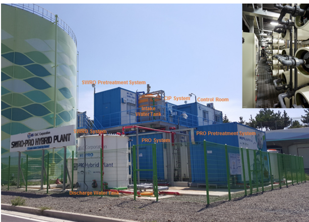
Fig. 8. SWRO-PRO demonstration plant located in a Busan wastewater treatment plant (240 m 3 /d, PRO system capacity).
