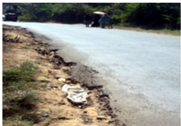
Fig. 2 Soft Shoulder Erosion at Mile Road in Bandarawela
