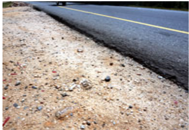
Fig. 1 Soft Shoulder Erosion in Kandy
