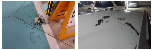
(a) Pollution of the floor of an underground parking lot (b) Pollution in the upper part (ceiling) of a car
