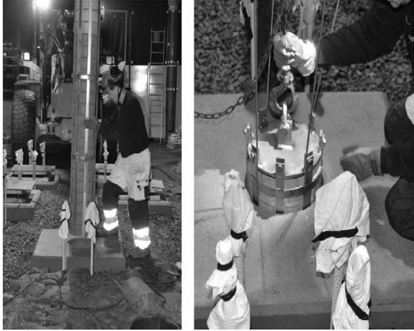
Fig. 12. Lowering the bentonite package into the deposition hole at the Aspö HRL.
