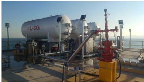
〈CO 2 injection facility〉
