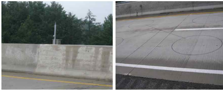
Fig. 10. Roadside weather measurement equipment and Contact type surface temperature sensor
