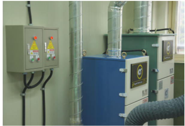
(a) Air cleaning system for vacuum assisted resin infusion facility
