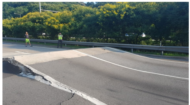
Fig. 1. Expansion Joint Damage 1) .
