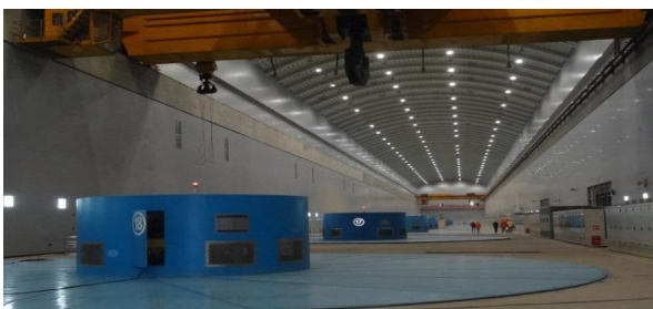
(b) 770 MW jumbo hydro-generators
