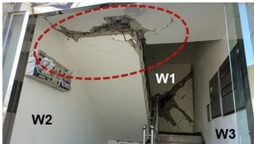
(e) Damaged stair case
