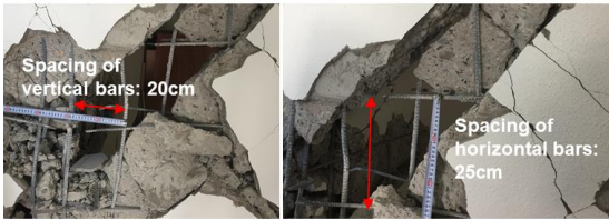
(c) Damaged wall W1
