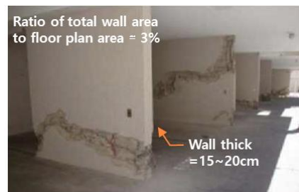
Fig. 12. Damaged shear walls in the first story in the 2010 Chile earthquake ( M_w 8.8) [16]
