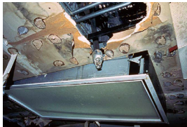
(a) Damage of sprinkler at new olive view medical center
