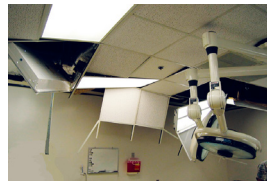
(b) Damage of ceiling at kona community hospital
