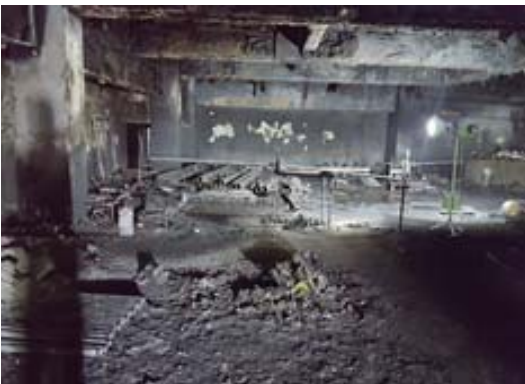
Fig. 1. The fire accident site.
