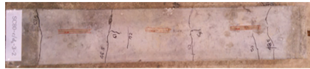
Fig. 12. Appearance of cracking occurrence
