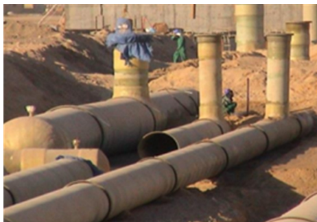
(a) Underground Pipes
