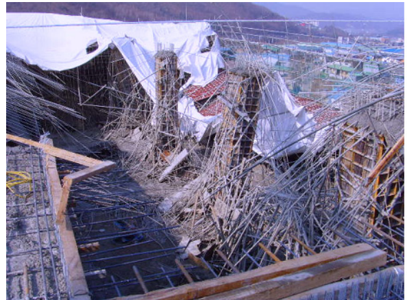
<Fig. 6> Storage construction accident
