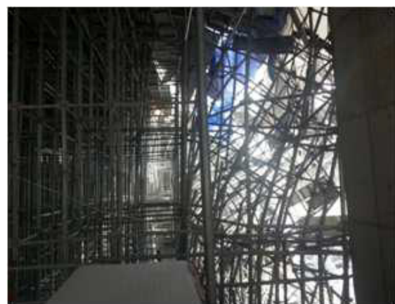
<Fig. 2> Cause of collapse (bracing not installed)
