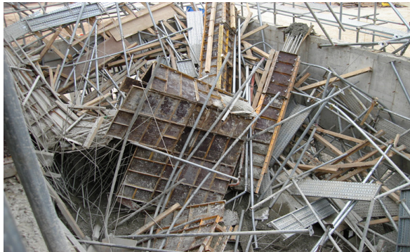
<Fig. 3> Collapse of system support during concrete pouring
