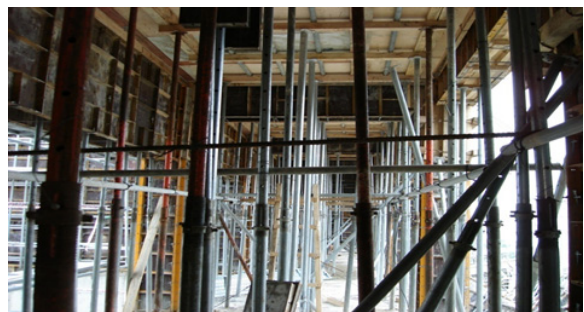
<Fig. 5> Violated horizontal member spacing criteria
