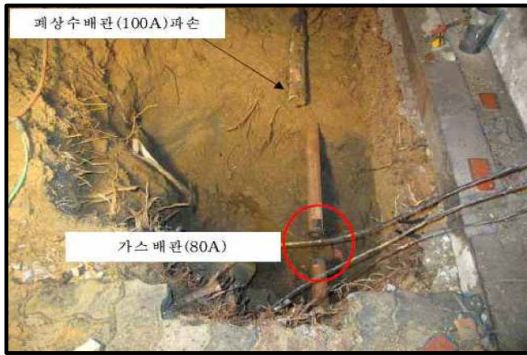
Fig. 1. Gas pipe exposed damage point and gas leakage fire point.[1]
