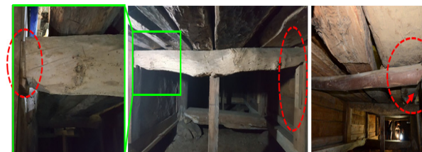
(c) Defection of wood plates sleeper No.4 and right wood
