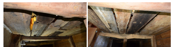
(e) Damage of top wood plates
