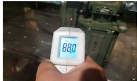
Fig. 8 Abnormal heat generations of the defective fuel pump
