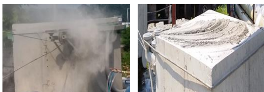
(a) Scattered dust during dry cutting (b) Remaining dust after dry cutting Fig. 1 Scattered dust and remained dust by dry cutting method
