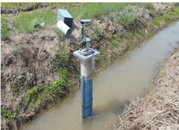
Fig. 1. Automatic water meter installed at the outlet of control(CT) block (Thalimedes, OTT, the Netherlands)
