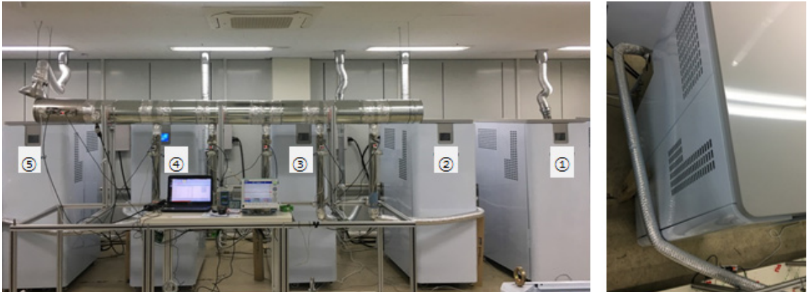
Fig. 4. Fuel cell system and common vent
