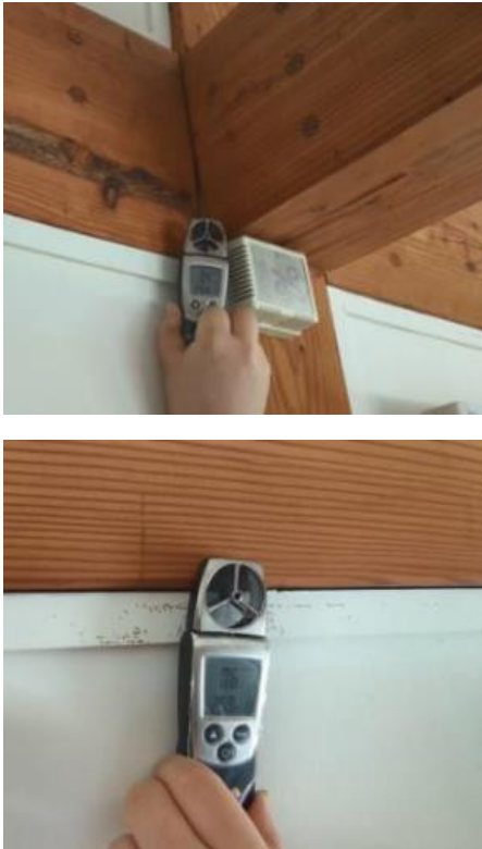
Fig. 8. Air leakage in post-beam construction.
