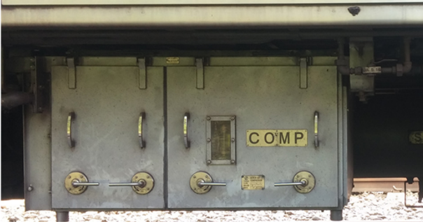
Fig. 3. Outside view of air compressor.
