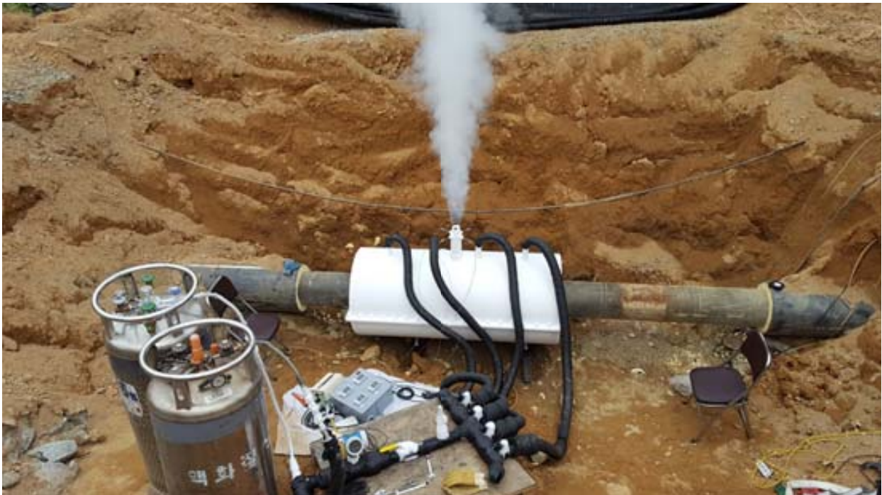
Fig. 6. Test of freezing seal isolation for pre insulated heat transport pipe(300A) at KDHC
