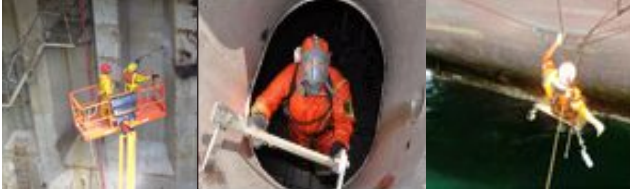
Fig. 1. Dangerous working conditions for maintenance/inspection.
