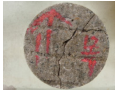
Photo 1 Pavement crack by AAR
