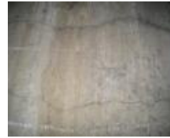
⑤ Abutment parapet crack
