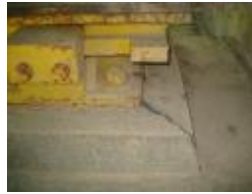
④ Shoe mortar crack
