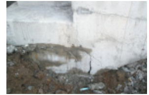
⑥ Abutment wing-wall crack
