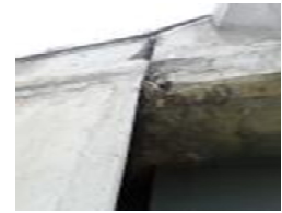
② Deck end spalling
