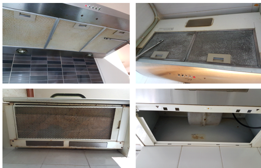
Fig. 3 Maintenance problem for Range hood
