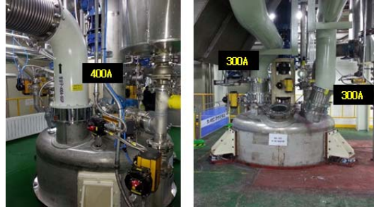
Fig. 7. The photo. of installed rupture disk on batch reactors.
