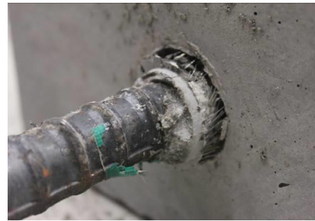
(a) Bond failure
