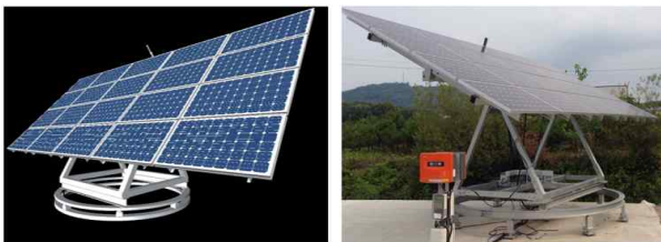
Fig. 10. 5kW solar tracker system
