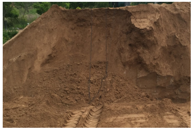
(b) slope failure (Case 2)
