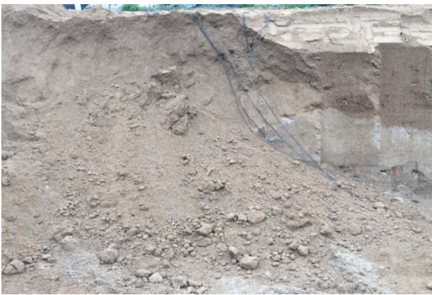
(a) slope failure (Case 1)
