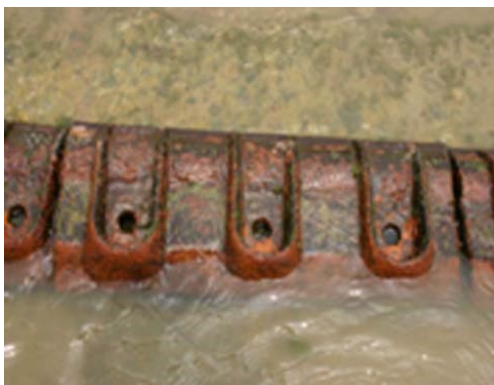
(a) Corrosion of steel clamping plate
